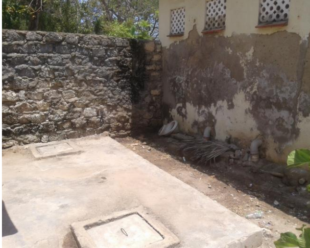
Plate 4-24: One of the toilets connected to a septic tank at Mwaepe Landing site belonging to one of the business owners on site
