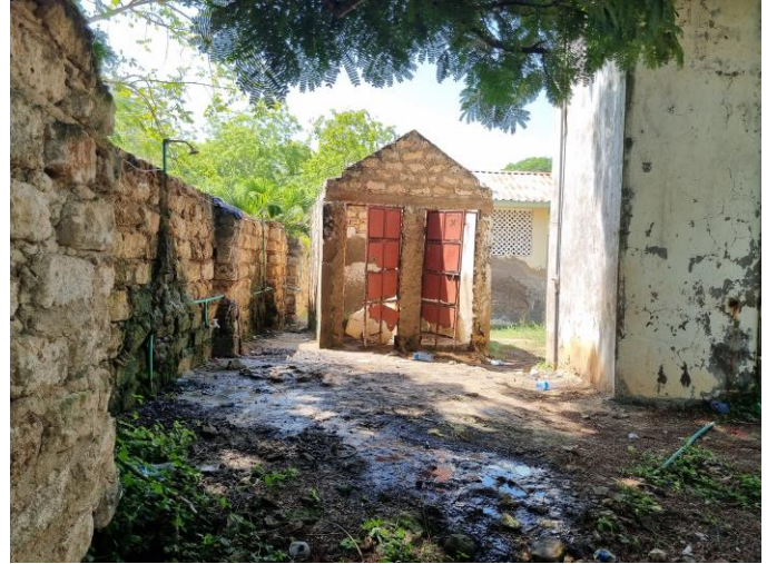
Plate 4-25: Dilapidated pit latrine used by fishers at Mwaepe site
