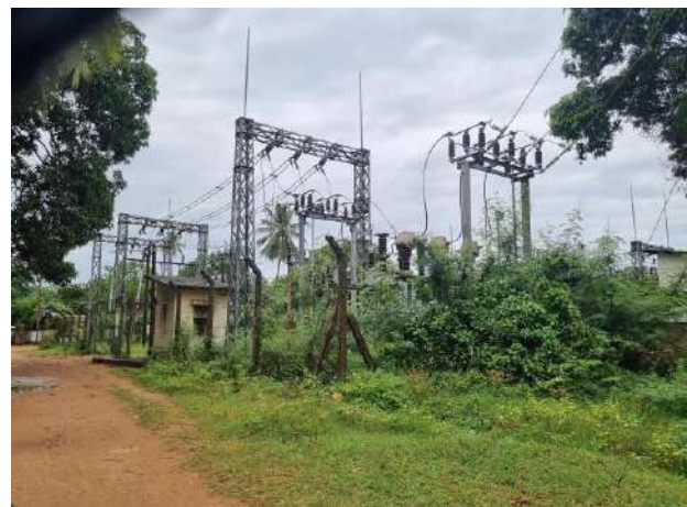
Plate 4-16: Power sub-station for supply of power within Msambweni area
