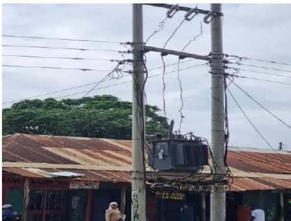
Plate 4-15: One of the Power Distribution Transformers in Msambweni
