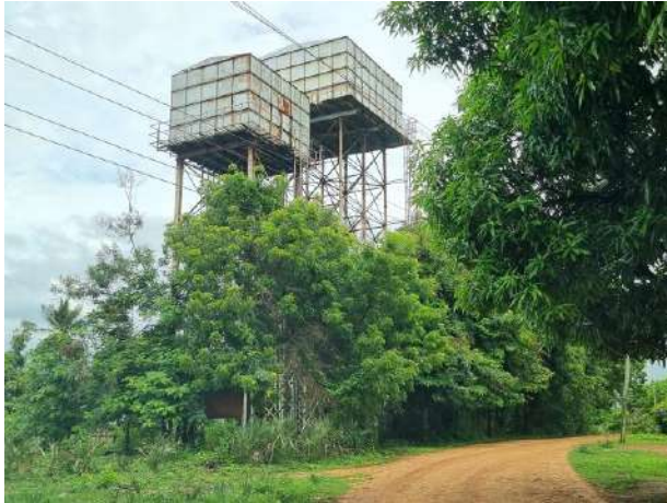
Plate 4-11: Elevated Steel Tank at Msambweni Referral Hospital
