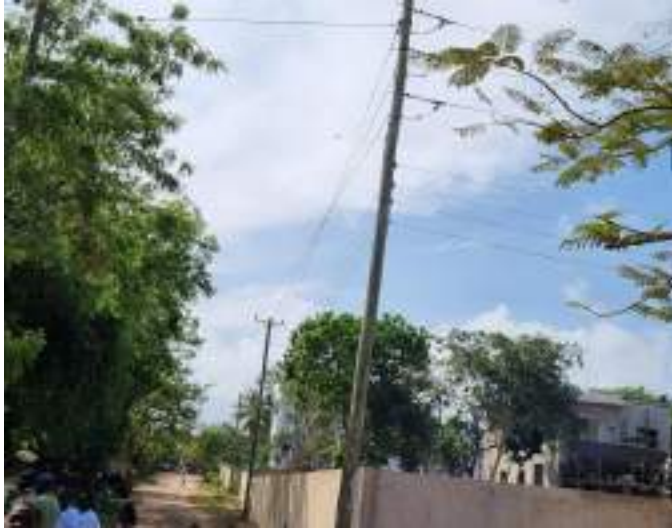
Plate 4-28: Power grid within the project site
