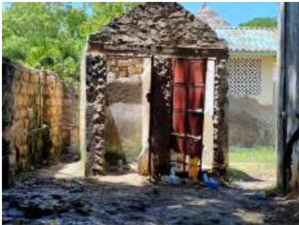
Plate 4-12: One of the sanitation facilities on site used by fishers in a bad shape
