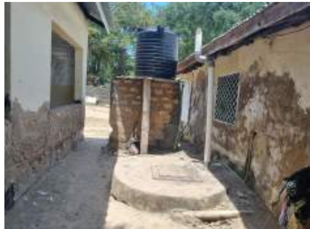
Plate 4-13: Dilapidated structures that are not pleasing to the eye on site
