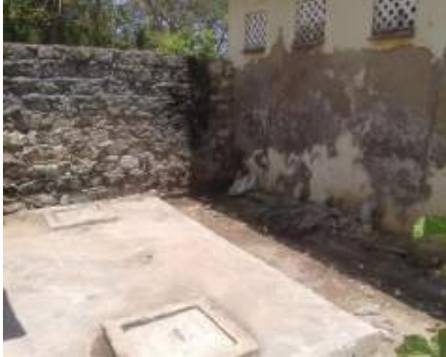
Plate 4-24: One of the toilets connected to a septic tank at Mwaepe Landing site belonging to one of the business owners on site
