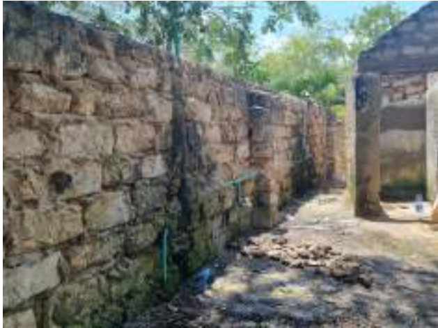
Plate 4-22: Part of the Water Piping System at the Landing site
