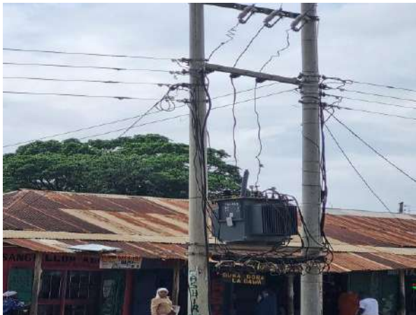
Plate 4-15: One of the Power Distribution Transformers in Msambweni
