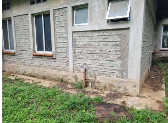
Plate 4-14: Connection of the existing offices in the plot to a septic Tank
